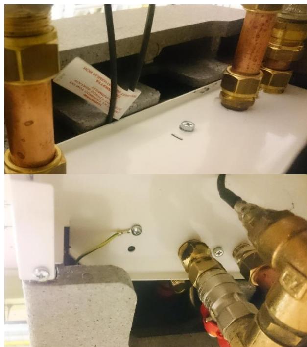
Figure 4 Non airtight 'insulating' substation cover, top in upper photo, underside in lower photo
